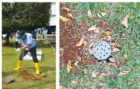
IEI employee digs hole for a biopore; a biopore in the ground
